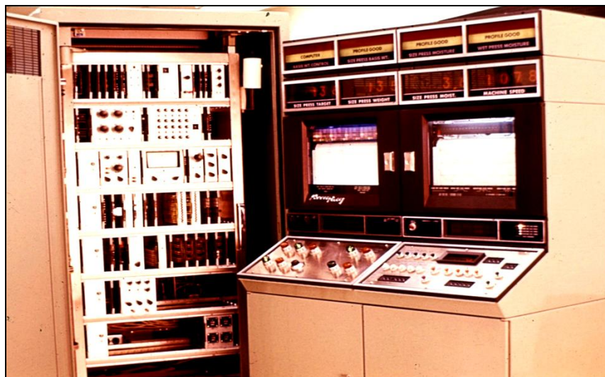
AccuRay 700 system (Remote cabinet with transistors & integrated circuits, Operator Console)
